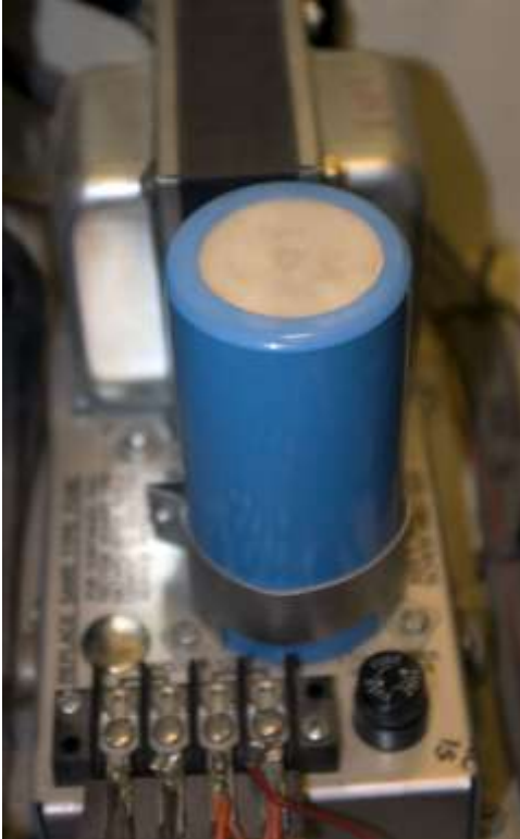
Figure 5 – Internal 12VDC power supply
